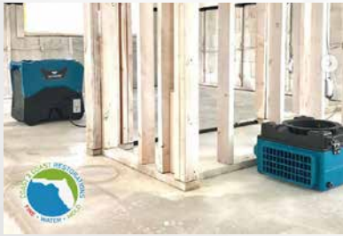
WATER DAMAGE RESTORATION
